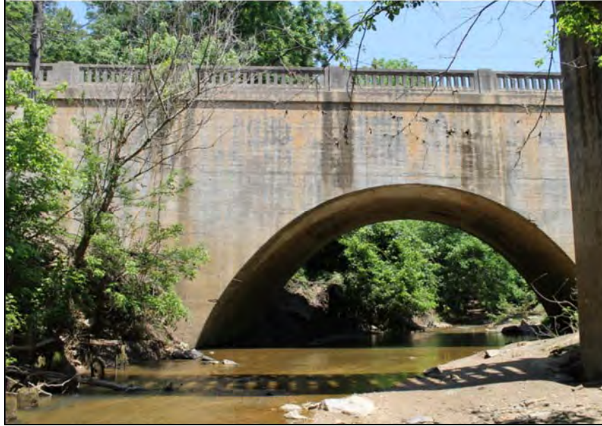
Figure 116: Bugaboo Creek Bridge, south elevation, photo graph by Royce and Bobette Haley, June 2017, accessed via https://bridgehunter.com/nc/wilkes/1930092/
